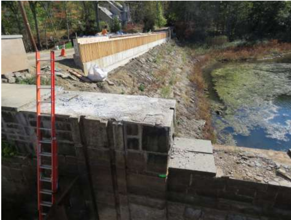
Capstone removal in preparation of right service spillway training wall removals for primary spillway expansion.
