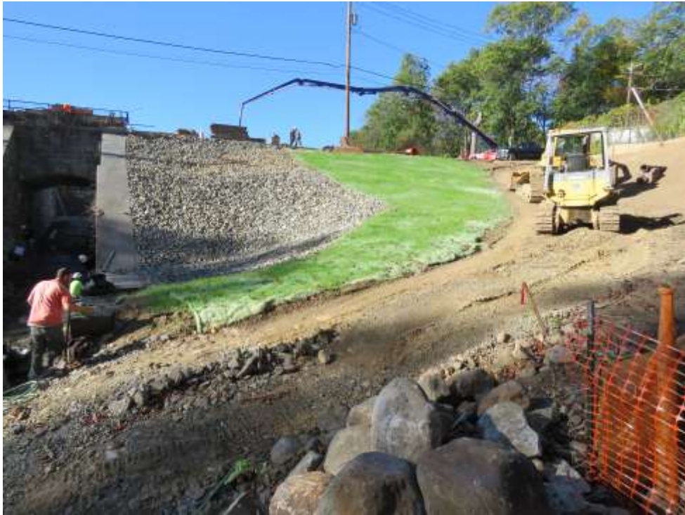
Left Side of Downstream Embankment Slope Showing completed rip rap and earth embankment. Permanent Access Road is not complete.
