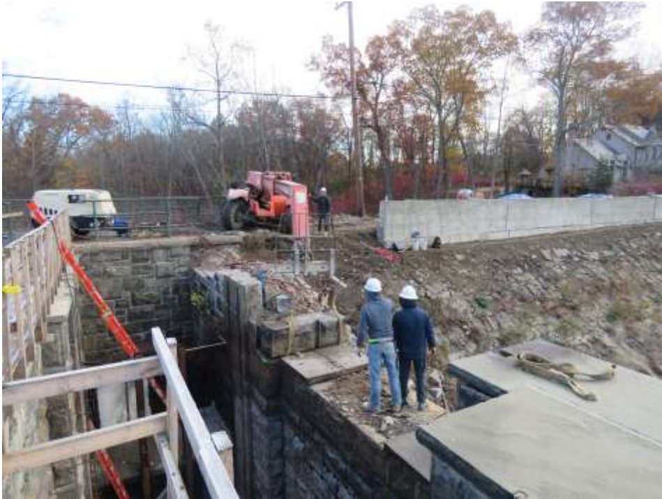
Primary Spillway, removal of existing stone masonry to expand spillway and construct forebay structure.
