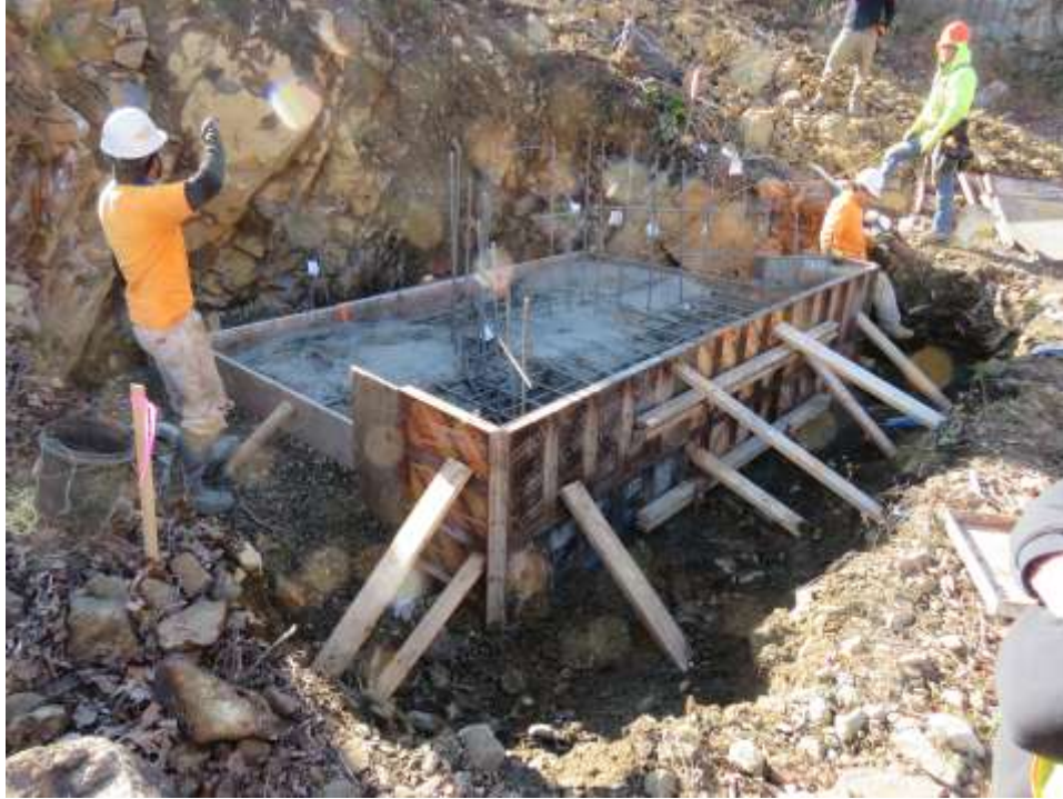
Construction of footing for LLO siphon system discharge structure at Pond No. 3. Photo shows shallow bedrock present within the right abutment.
