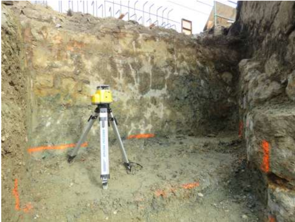
Excavation of re-entrant corner on left side of auxiliary spillway. Photo shows stone masonry corewall.
