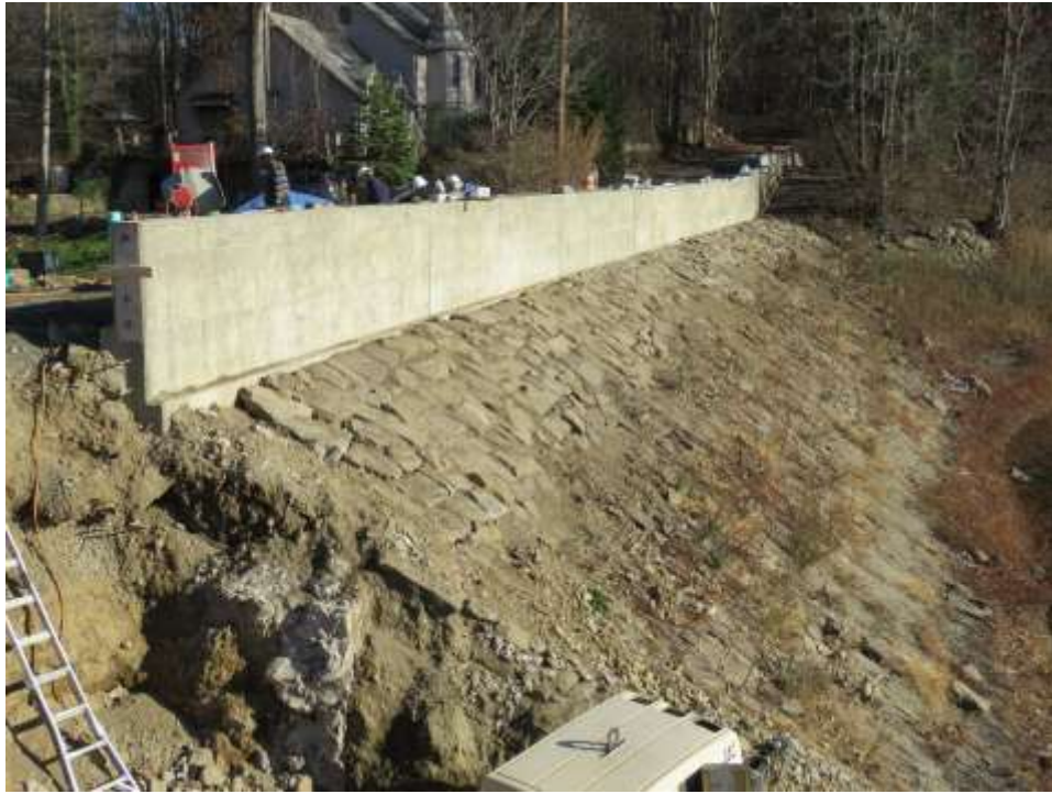
Completed armoring of u/s embankment slope along parapet wall Segments D and E.
