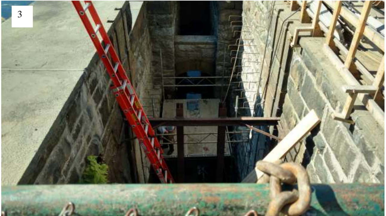
Service Spillway showing installation of grouted dowel hooks for overpour concrete wall construction.
