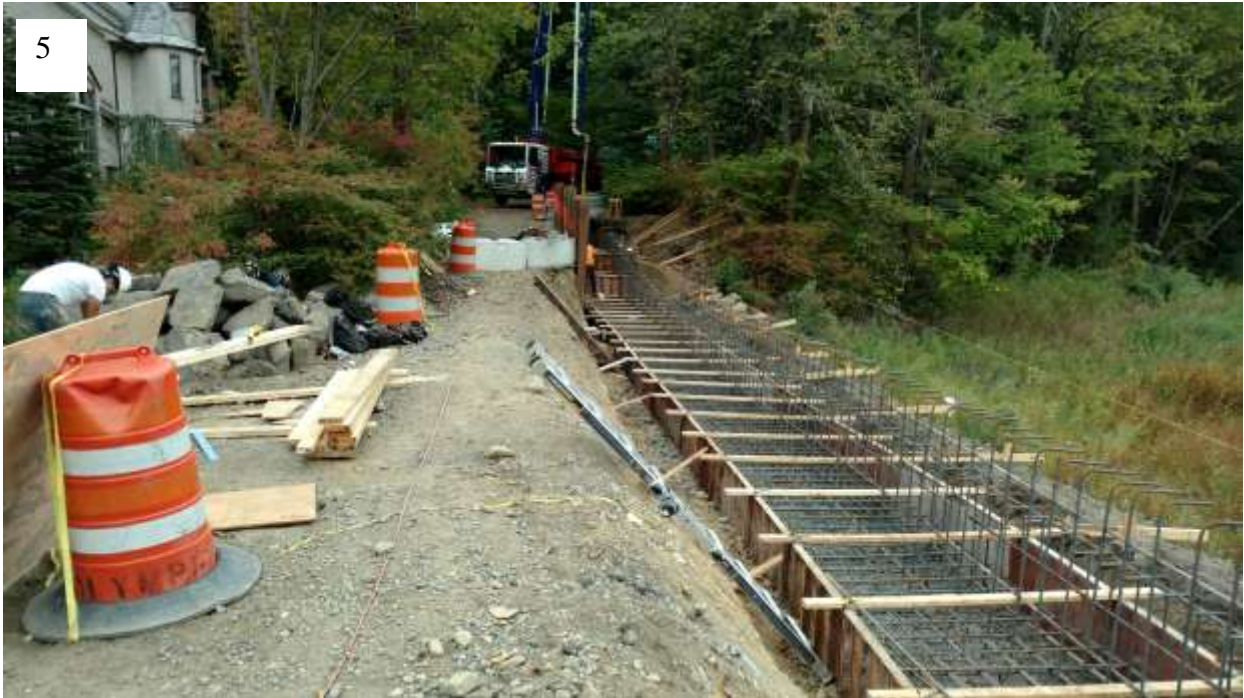
Start of parapet wall base construction. Note concrete pump truck at east end of the wall.
