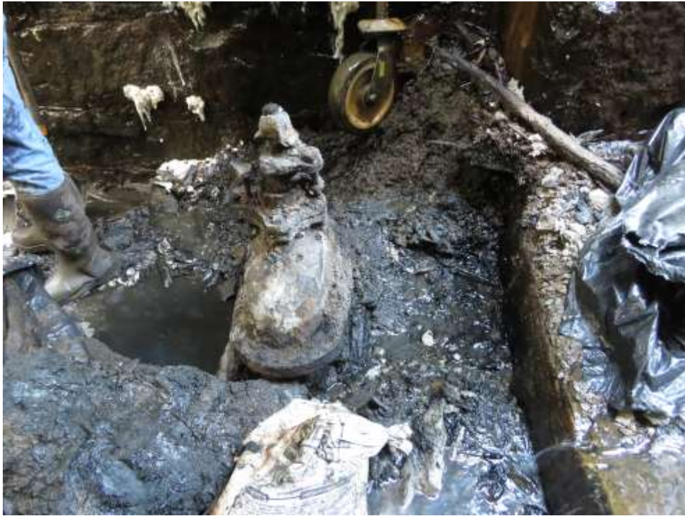
Outlet Valve within Service Spillway Sump.
