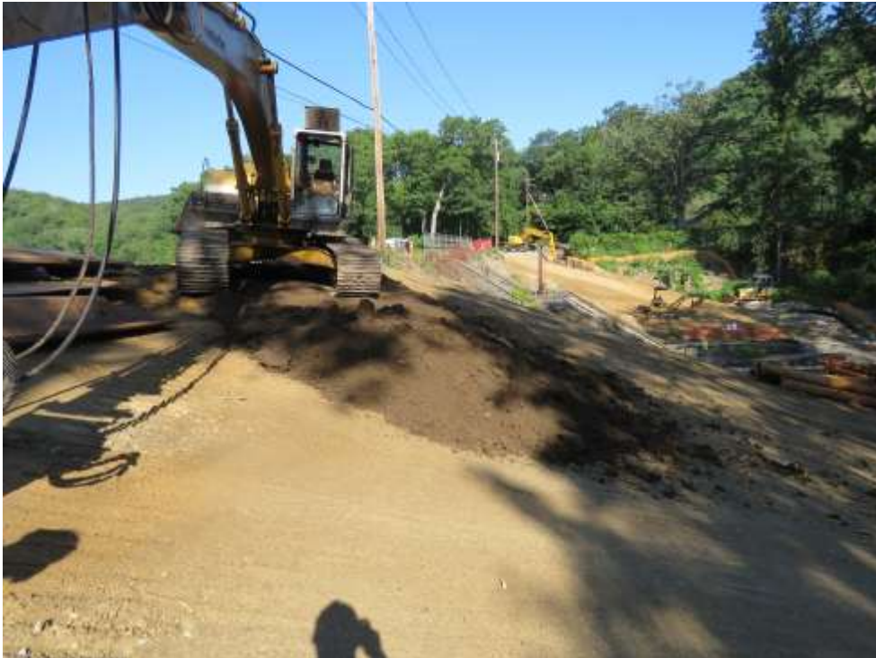
Right Side of Downstream Embankment Slope with Topsoil being stockpiled. Pipes shown (right side of photograph) are abandoned pipes removed from the service spillway discharge channel.
