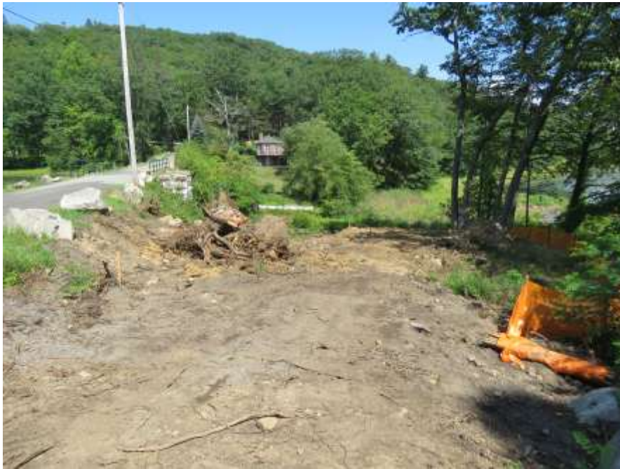
Pond No. 3 stump removal and clearing and grubbing of LLO siphon trench alignment.
