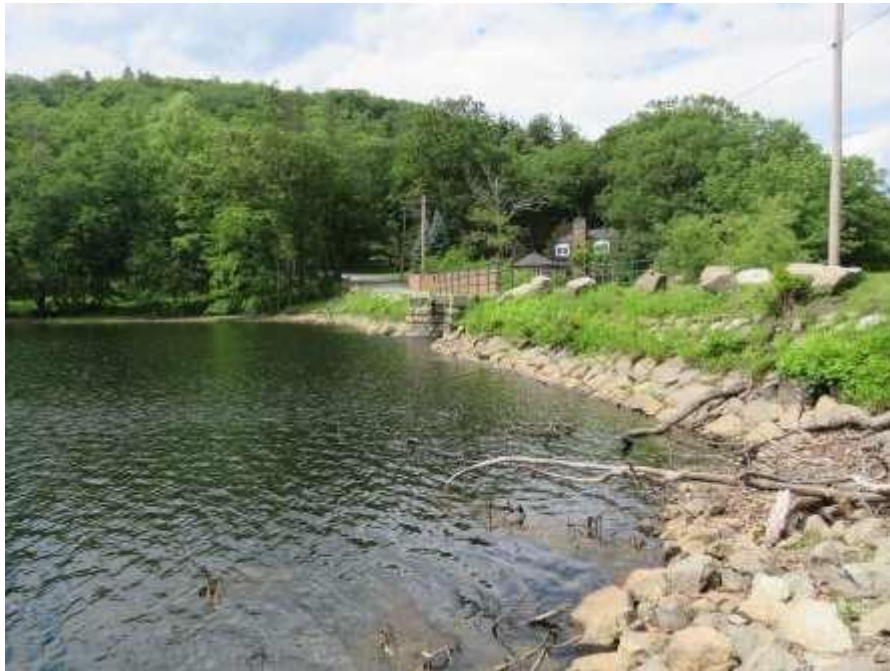
View of Pond No. 3 at Construction Pool. Dam Repairs and Modification Anticipated for Late Summer.
