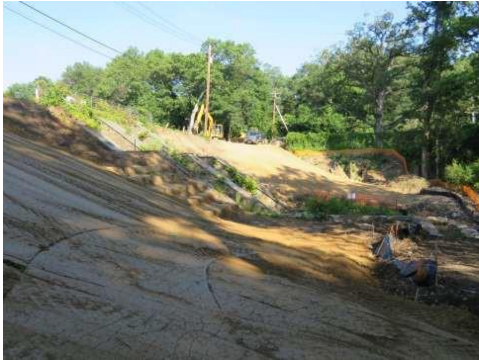
Compacted Embankment Filled on right Downstream Slope after Sealing with Compactor ahead of rain.
